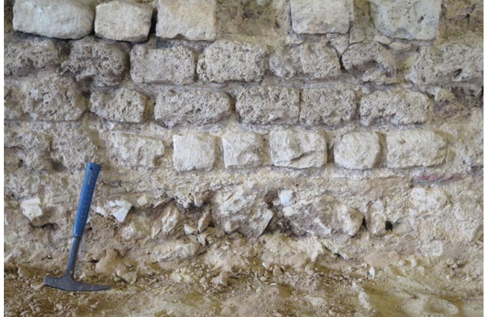
Figure 8.21 Piece of ashlar from the southern wall of the bathhouse, consisting of cut blocks of Kunrade stone (white) and sawn blocks of porous calcareous tufa (beige) over an inner wall of rough blocks of Kunrade stone (source: R. Dreesen).
