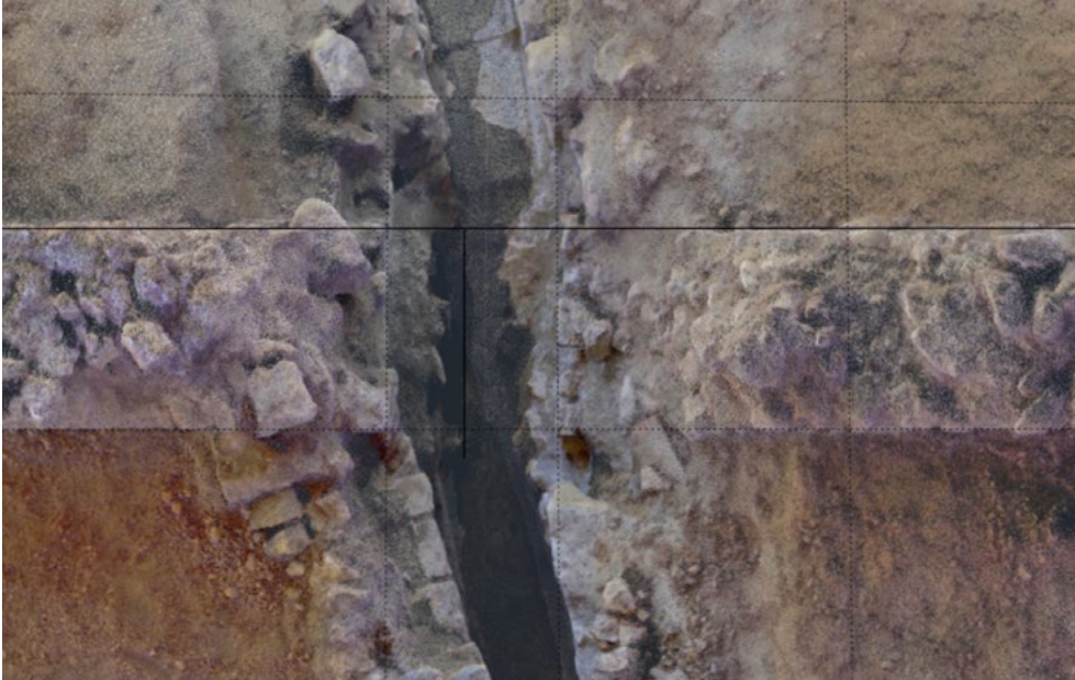
Figure 4.21 Original and secondary opening for the main drain through the south wall of the portico (source: Delfttech/K. Peterse).
