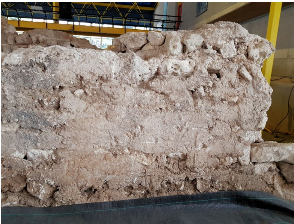
Figure 4.12 The mortar in the west wall of praefurnium I is also found on the wall surface, where it has seeped out into vertical, more or less smooth patches. This suggests that this part of the west wall was built against the vertical cut into the soil, which served as casing for the wall (source: K. Peterse).
