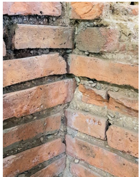
Figure 4.9 Tegulae used as bricks extend alternately from one wall into the other, showing that both walls belong to the same phase of construction (source: K. Peterse).
