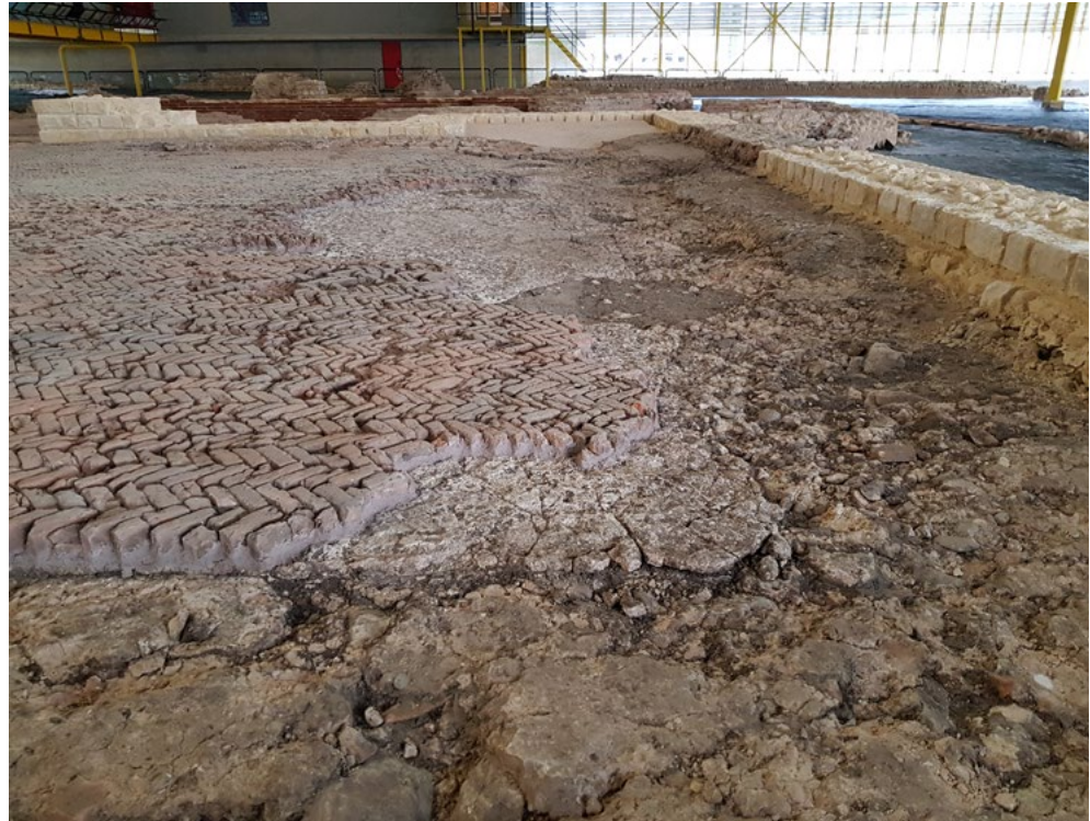
Figure 4.3 The westernmost part of the floor of the apodyterium has subsided substantially (source: K. Peterse).
