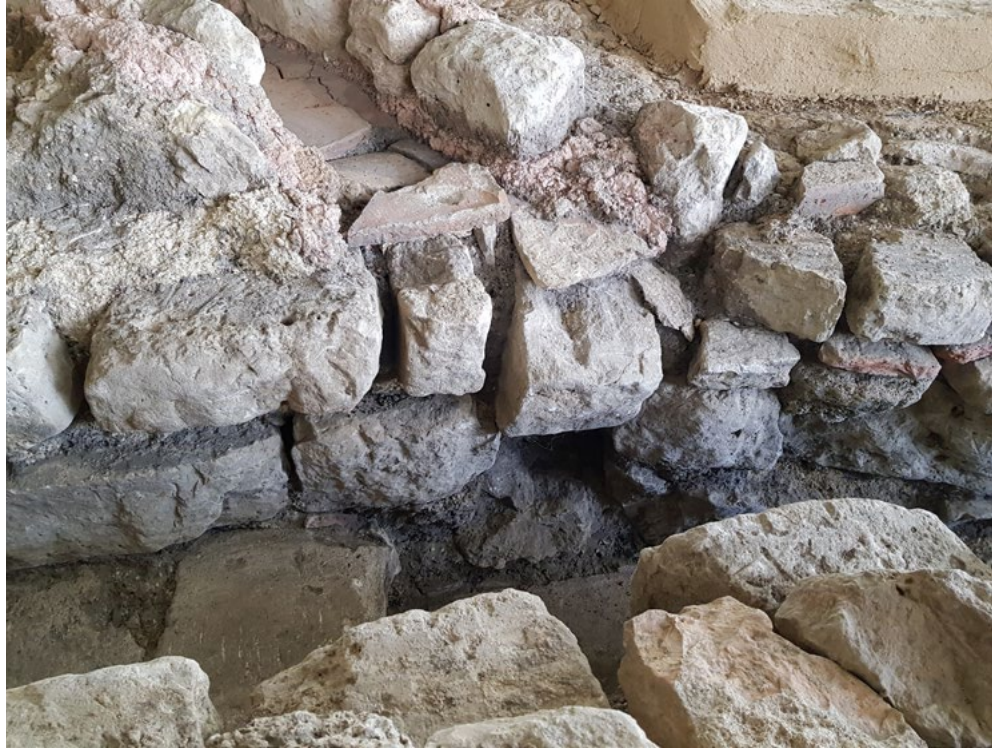
Figure 4.20 Transition in the main drain from the relatively shallow to the deep section, into which the drain of the natatio most probably emptied (source: K. Peterse).
